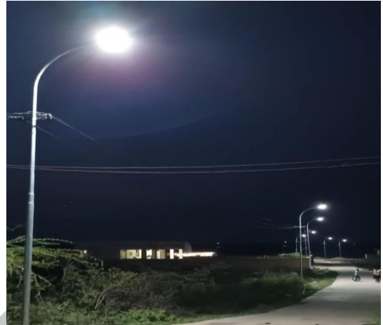
Streetlight at Khan Ki Jhopadiyan
